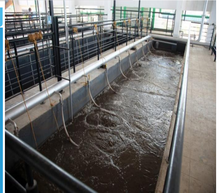
Sewage treatment plant with MBR technology
